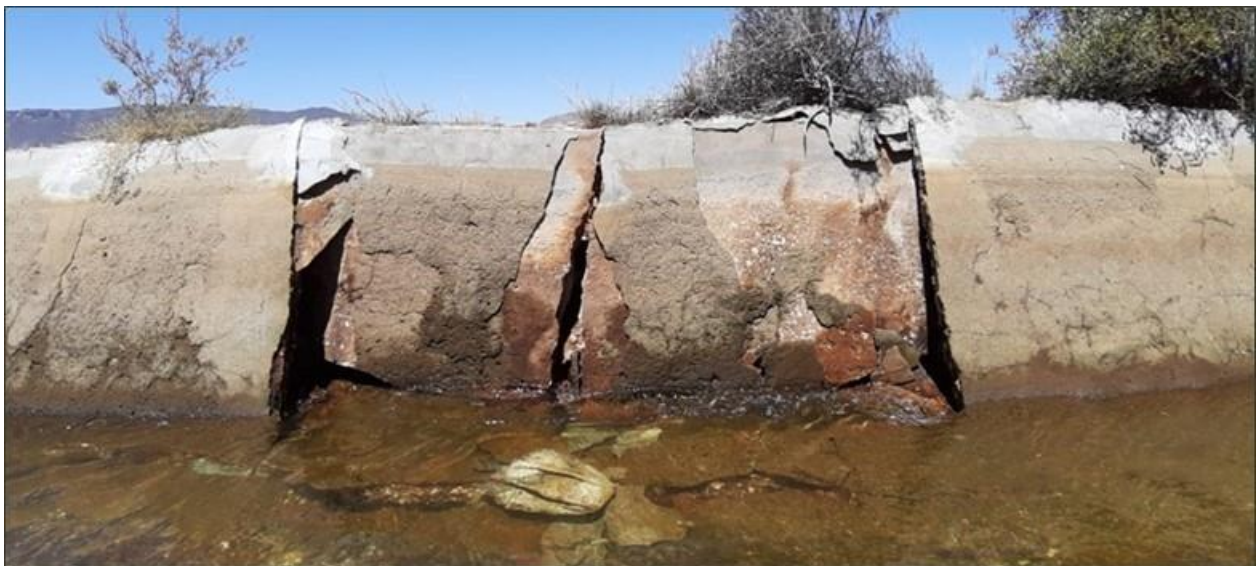
Figure 5.1: Failure of the Lower Olifants Canal along the main (Trawal) section
