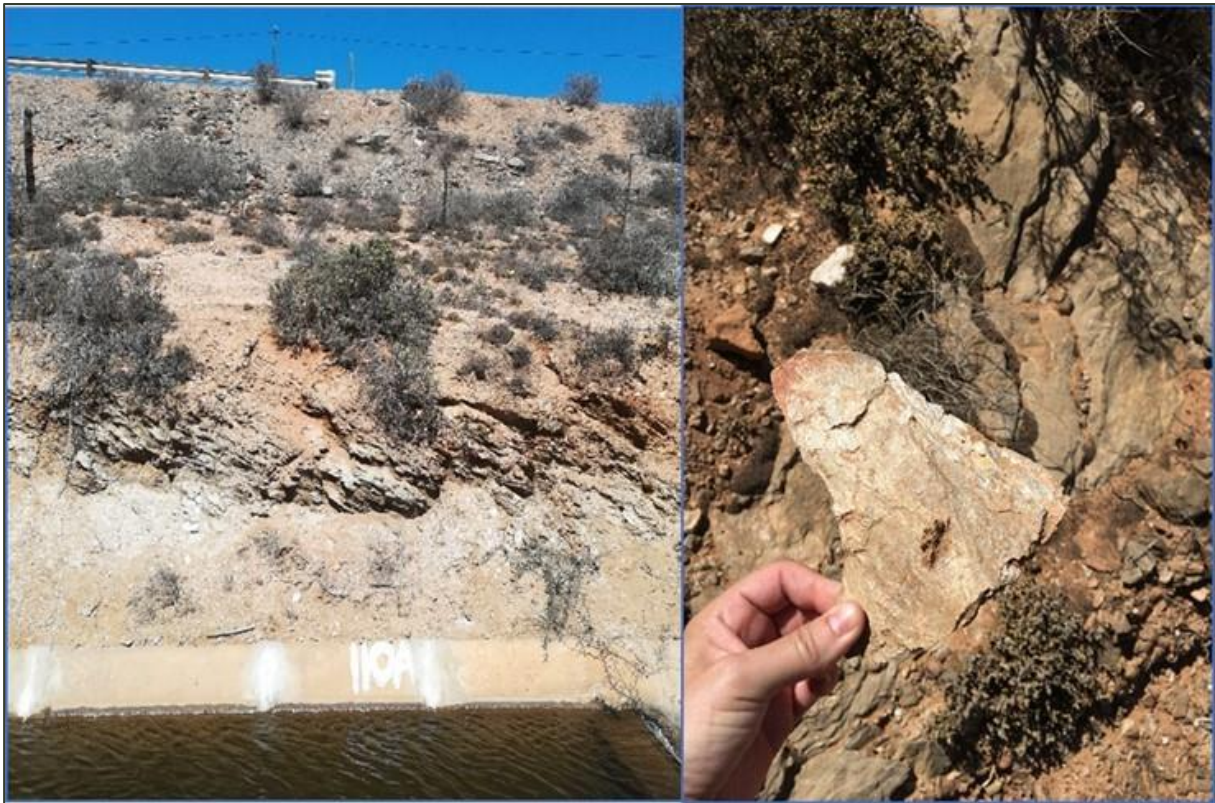
Figure 6.11: Exposed phyllite dipping at 40° towards the South-East
